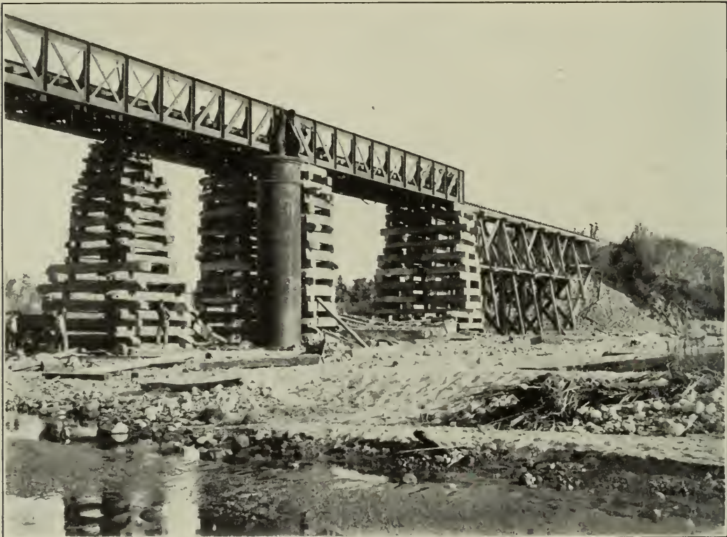
BRIDGE ON MANILA & DAGUPAN RAILWAY, DESTROYED BY INSURGENTS AND PLACED IN CONDITION FOR TEMPORARY USE BY ENGINEER TROOPS.
